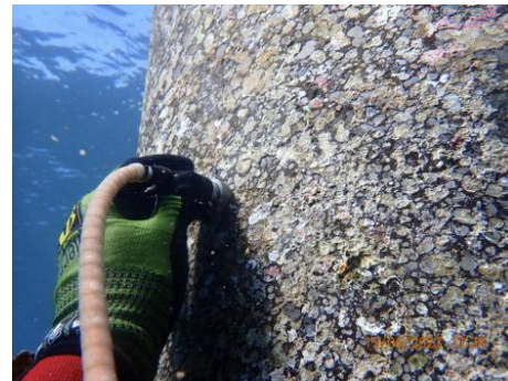
Photo 4 Example of Underwater CHS Condition
