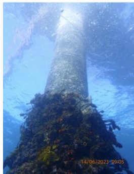
Photo 3 Example of Underwater CHS Condition
