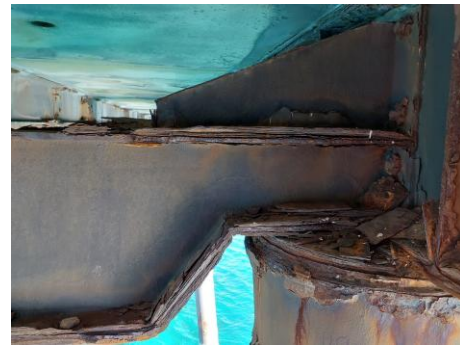
Photo 2 Example Photo of CHS Corrosion at Primary Beam Interface
