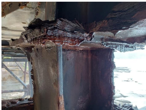
Photo 8 Example Photo of Deteriorated Connection
