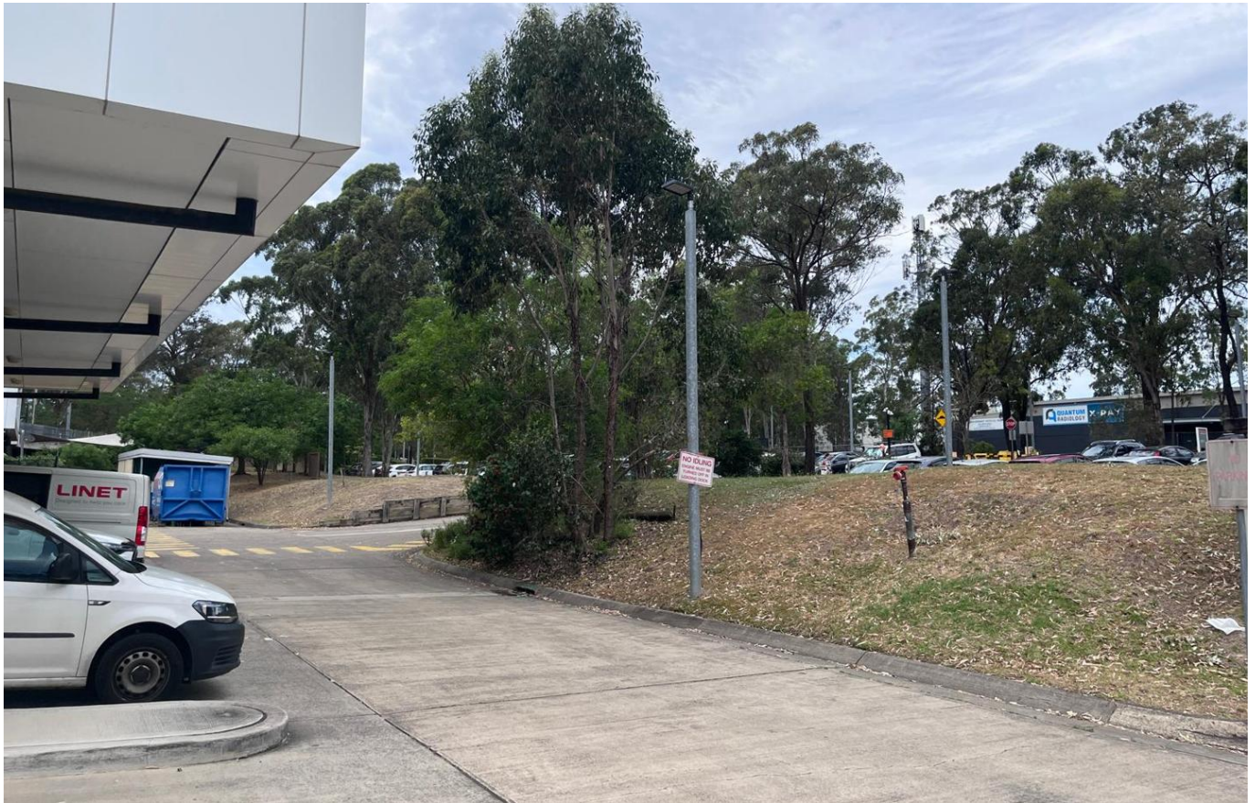
Figure 15 - Back of house and loading dock area and location for part of new fire hydrant ring main
