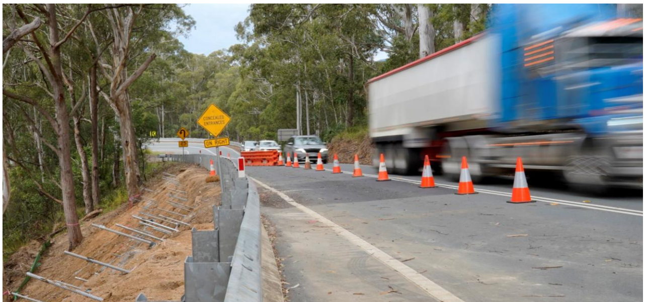
Figure 13. Slope repairs on Snowy Mountains Highway at Brown Mountain following floods in 2022
